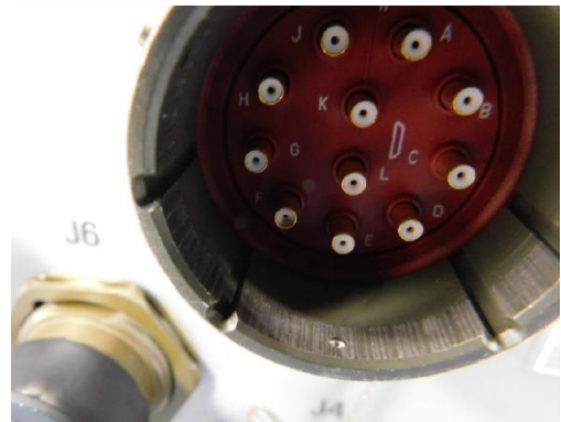
Figure 13: the IPT identified a trend in failed connectors and were able to immediately adjust and adapt so that a timelier repair option was available.
